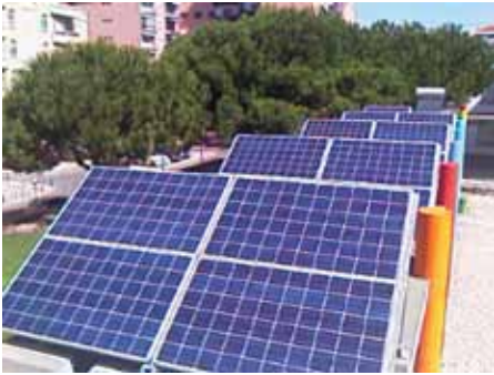
Educational center with renewable energies TORRES VEDRAS, TOWN HALL
